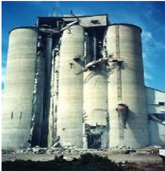
Figure A.1. Failure of grain silo, (dust explosion).
