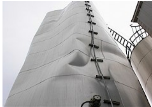
Figure A.6. Failure of steel silo, implosion.
